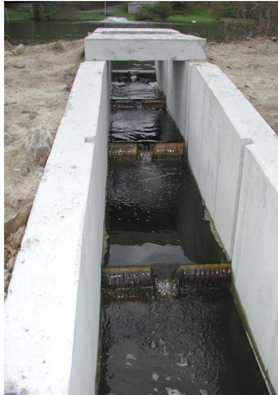
Lake Tashmoo Control Structure/Ladder
